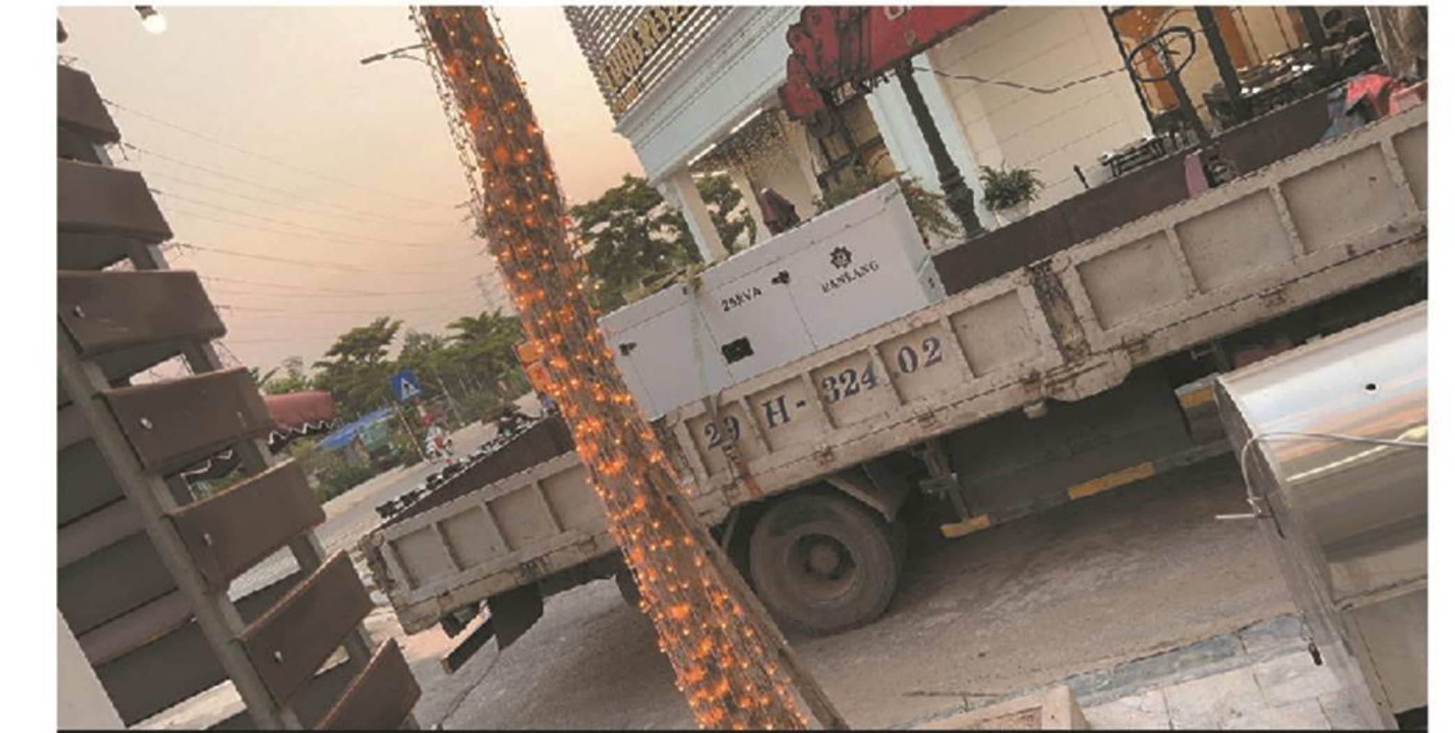
Hanoi Thien Nghia Restaurant YIQI 20kVA
